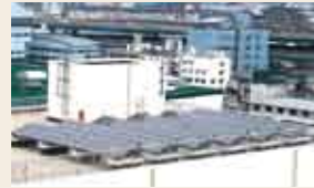
Solar panels on roof of Higashi-Nada Plant
