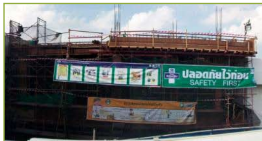
Prepared mix products productivity expansion construction at Thai Nisshin Technomic Co., Ltd. (Thailand)
